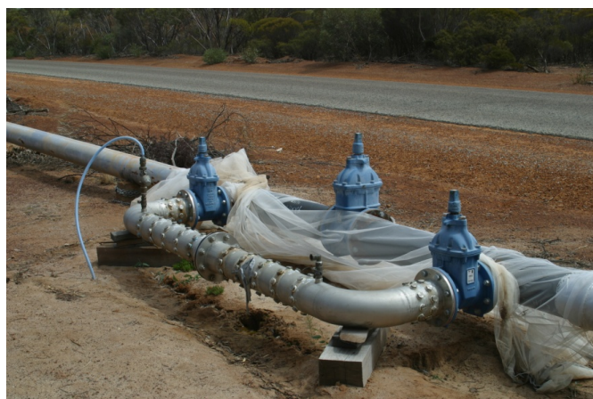
Figure 4: Modified Robbins device in water pipeline for biofilm research
